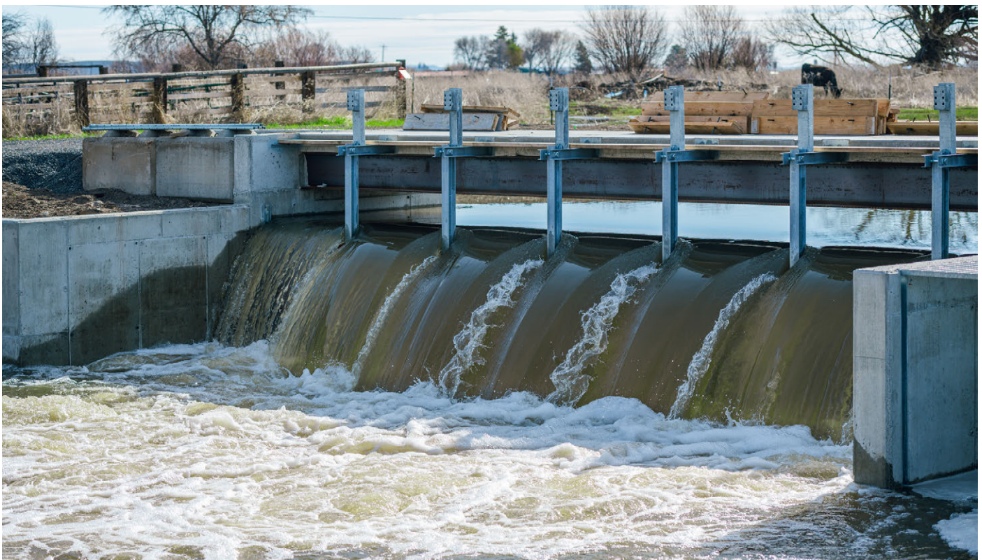
The new Sweek Dam along the Silvies River completed fall of 2019. Photo by Jeremy Hill, jhillimages.com.
