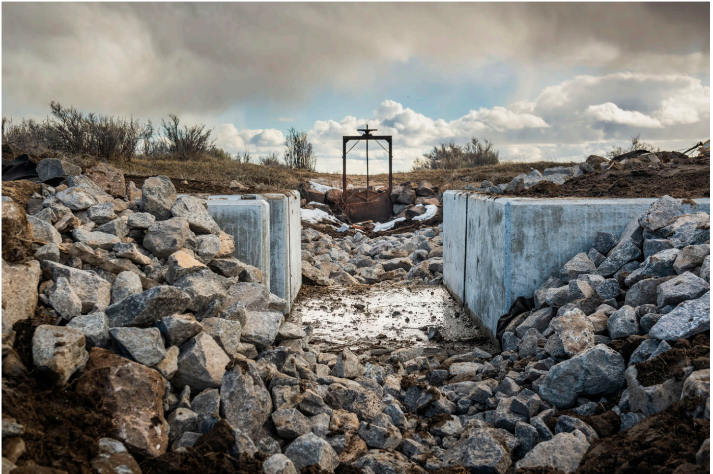
A new concrete diversion structure to more effectively move water to the head gate in the distance. The head gate can be opened as needed to flood the meadow with water that lies beyond the gate. Photo by Jeremy Hill, jhillimages.com.
