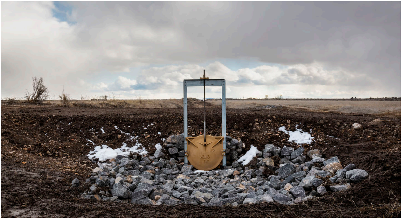
At the LY Ranch on the edge of Burns, OR wild flood irrigation infrastructure improvements were made, like the addition of this new headgate, to better manage water flow and irrigate fields that previously were not able to be irrigated.
