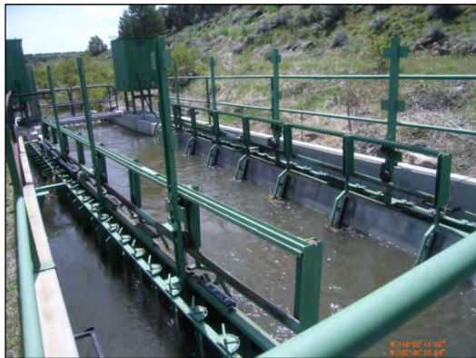
Figure R-19. Operating fish screen on the West Canal at Page Springs Dam.
