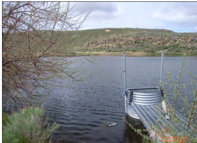
Figure R-18. A water control structure at Barn Yard Spring in the Double-O Unit.
